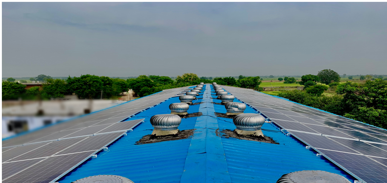
Our Green Initiative: 100Kw Solar Plant Commissioned in 2019
